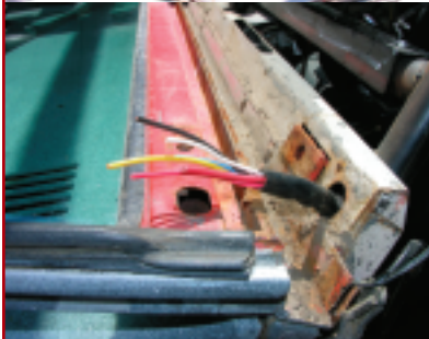
2. The first task is to remove your old frame. This can be easy to hard depending on your top, how many Bronco accessories you have added, and how many years of rust are holding things together. One thing everyone will need to do is carefully expose the existing wiper wiring running to the top mounted wiper motor and move it safely out of the way for later rewiring.
